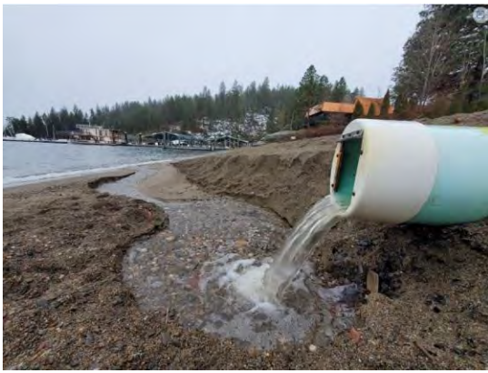
Figure 7. Uncontrolled stormwater outflow causing beach erosion.
